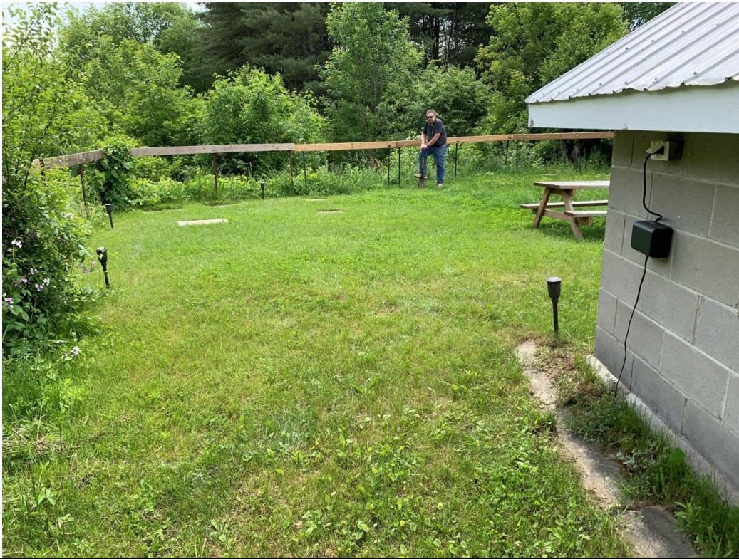
Haven mosquito repellent system being installed by Gordon Webster on the south mound, June 2022
